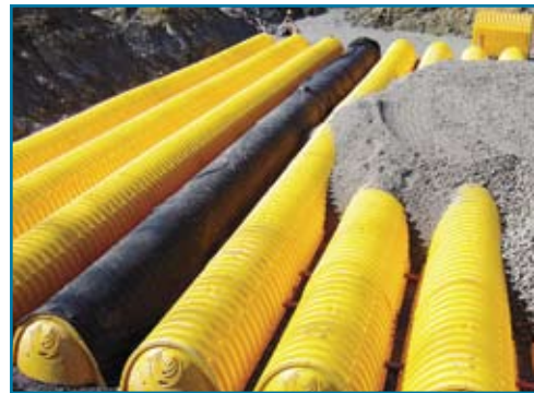
Isolator Row Technique Used To Enhance Total Suspended Solids (TSS) Removal and Provide Easy Access for Inspection and Maintenance.
