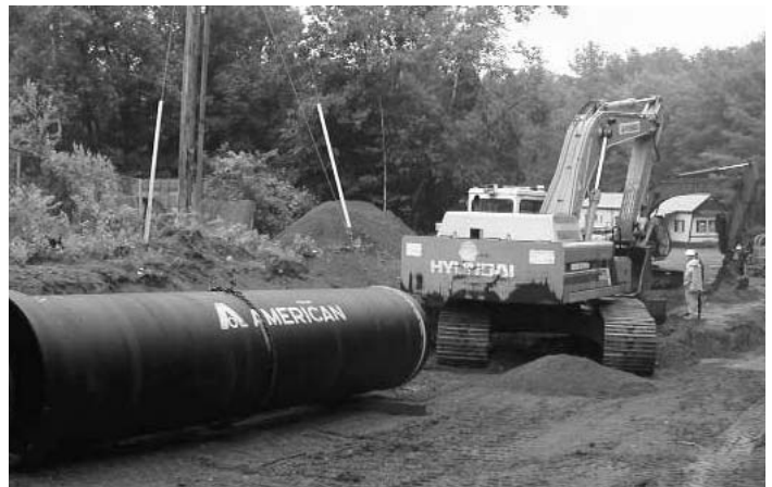
QWP and ACIPCO teamed up to supply the necessary equipment for the recent upgrade to the Hartford, VT, Water Treatment Plant.
