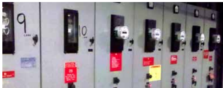
Some of the new FlexNet™ meters already installed.
